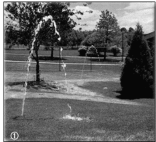
These sprinklers have broken heads, therefore creating a lawn fountain and water puddle.
